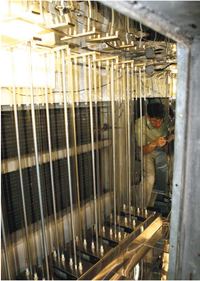
Figure 3. UVGI installation (turned off). Lamps are oriented vertically; reflective sheeting increases UV reflection from plenum walls.
