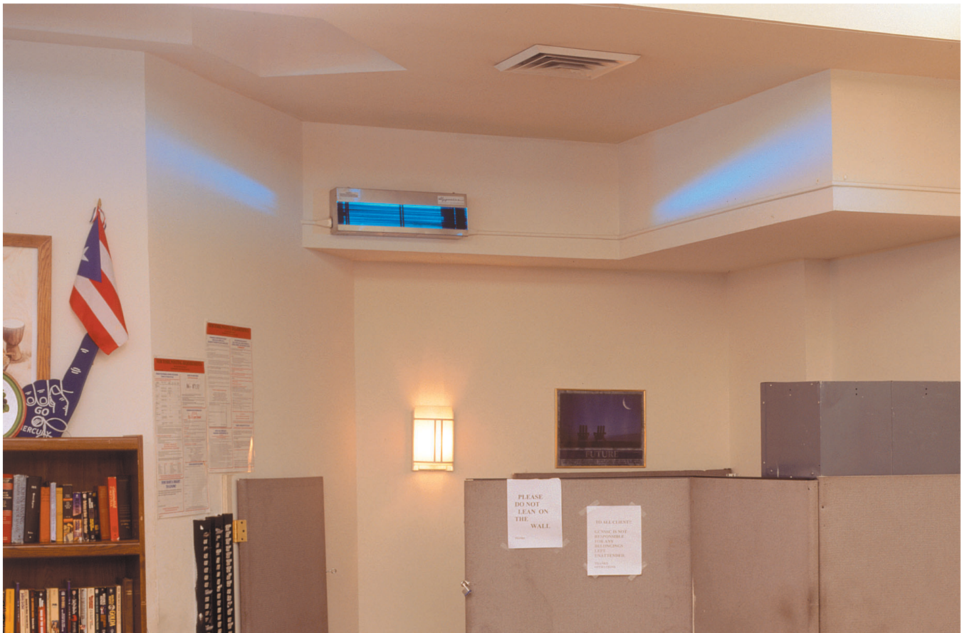
Figure 7. A wall-mounted UVGI fixture used in the St. Agnes Shelter for the Homeless (the distribution of ultra-violet radiation from the fixture is indicated by the pattern of blue light on the nearby walls)
